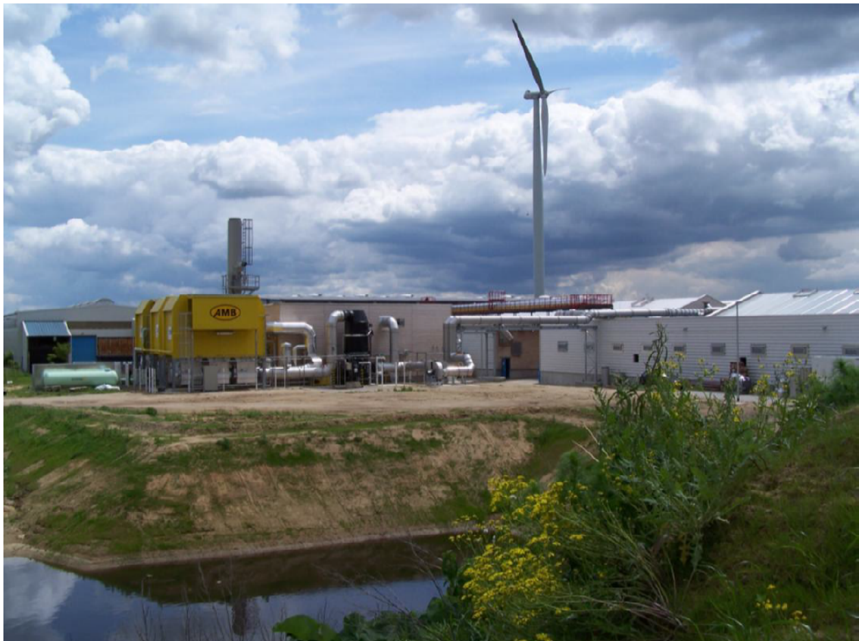
Figure 1 Expanded MBT Schwanebeck, view on exhaust air cleaning facility
